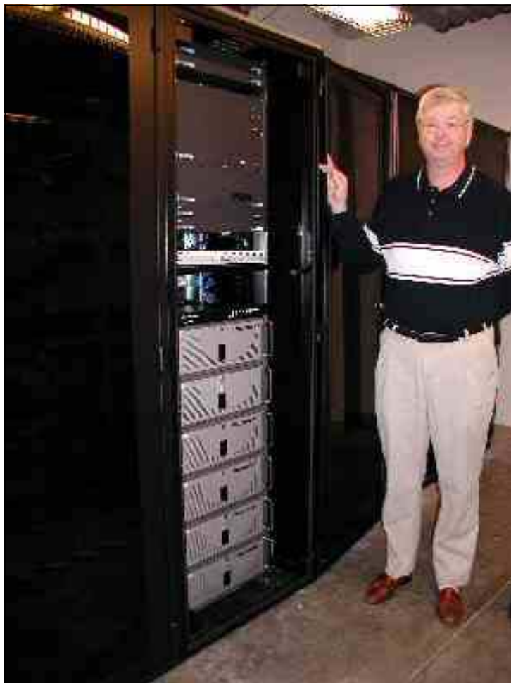
Larry Heilman, president of Smith Audio Visual, oversaw the replacement of the security system's timelapse video recorders with a matrix of five Crest CDVS-5416-240 digital video recorders, fed by a mixture of Pelco PTZ, Crest CJ-9124 and PRI 950P3 cameras.
